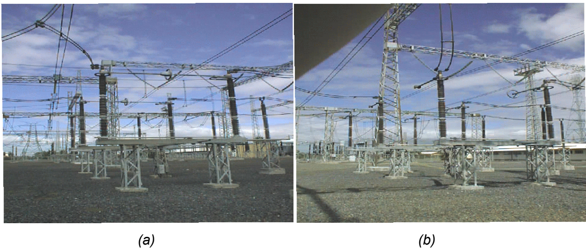
Fig. 1.31: Typical rotating arm isolators: (a) Isolator closed and (b) Isolator open.
